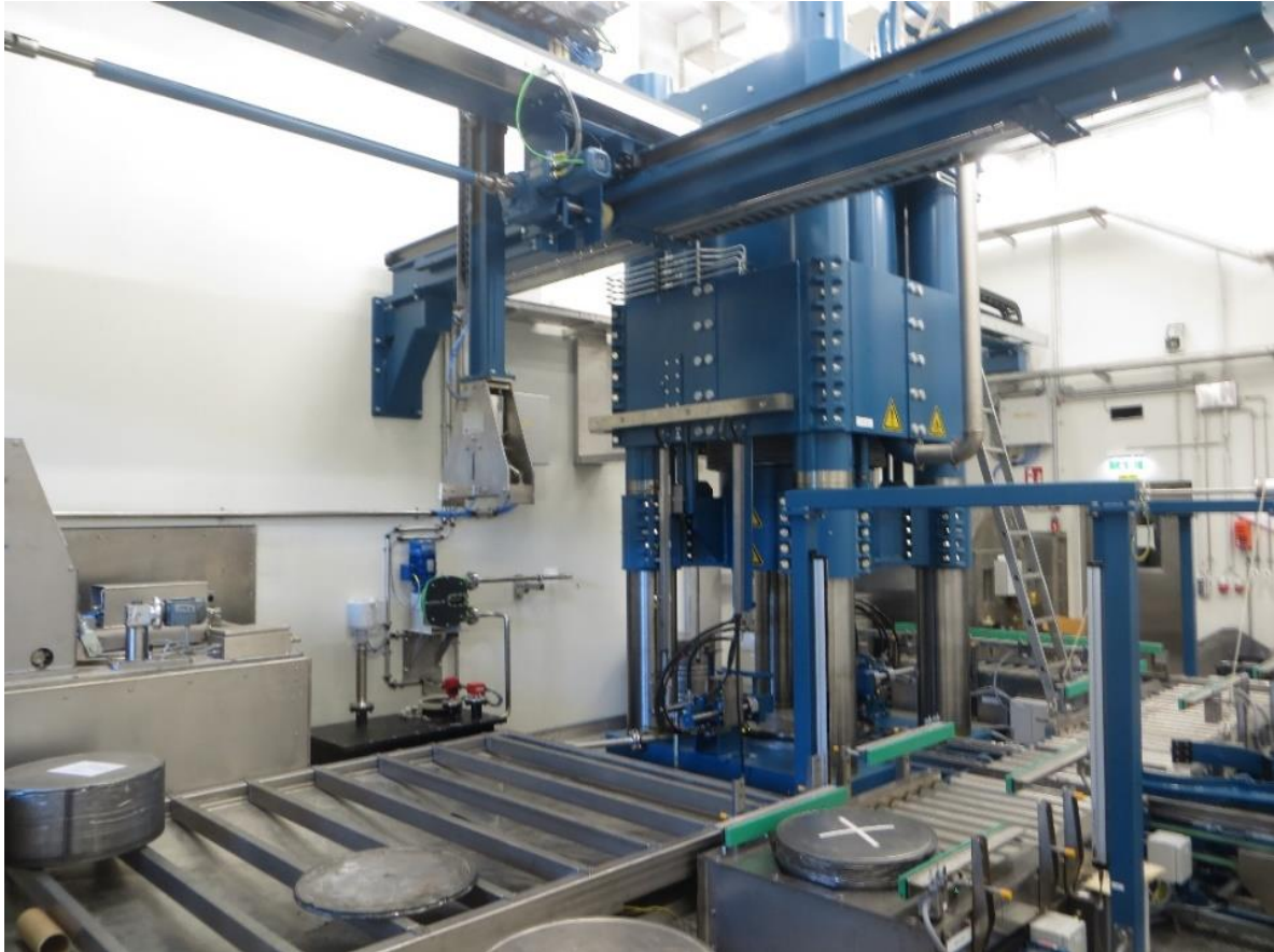
Figure 3 New super compactor with parts of handling system, © NES
