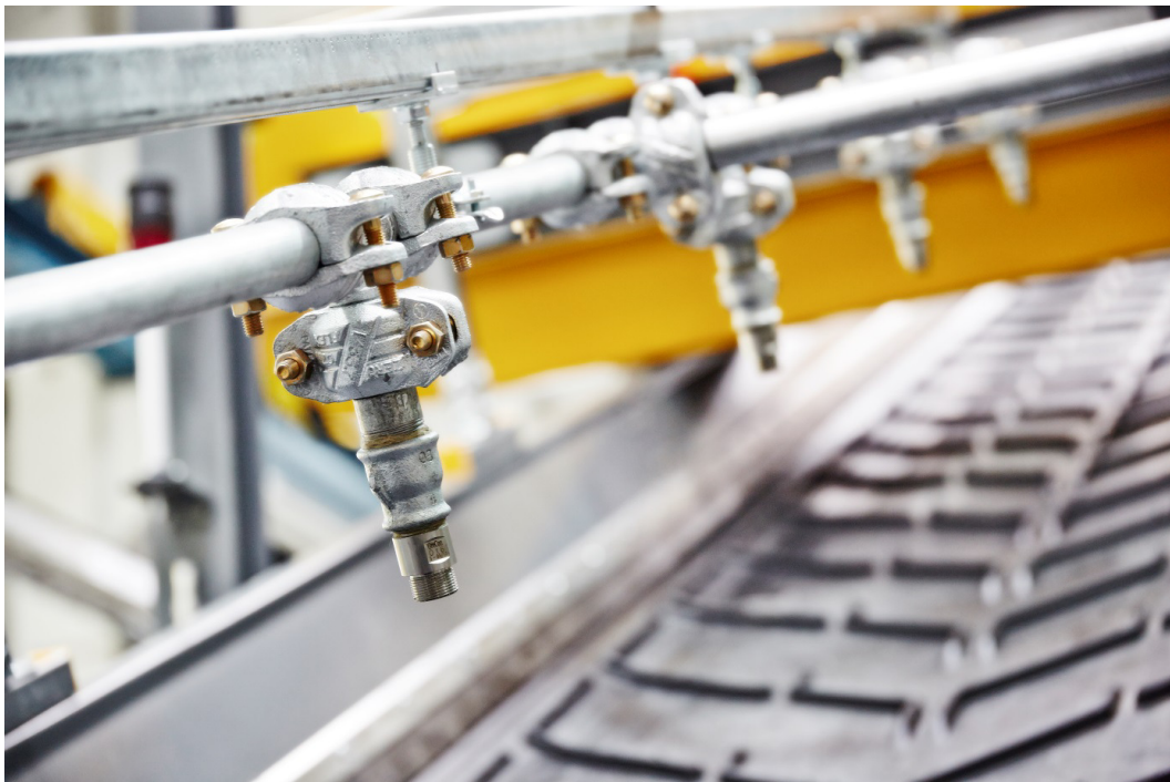
Example of state of the art automatic, quick-reacting extinguishing system
