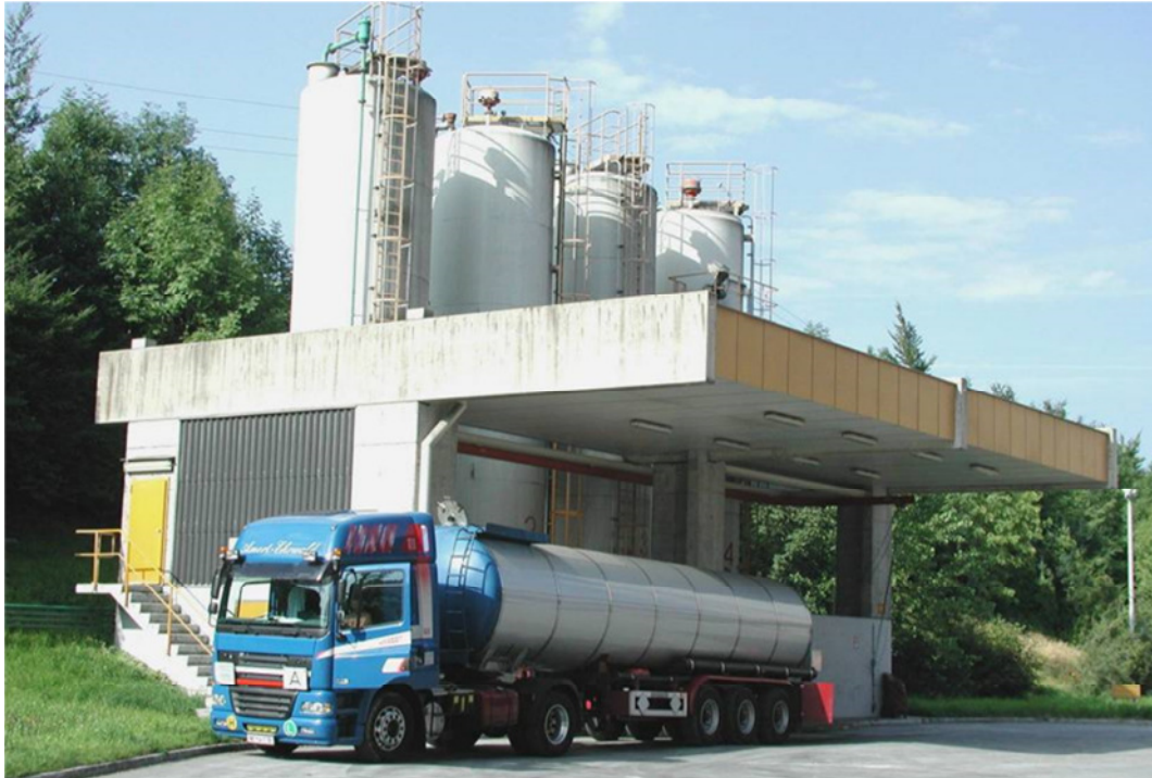
Station for reception of waste oil and non-halogenated organic solvents for thermal treatment at the cement plant in Gmunden
