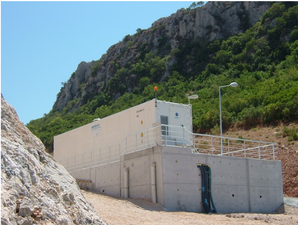
Treatment of 60 m 3 /d leachate in reverse osmosis plant in Kusadasi, Turkey
