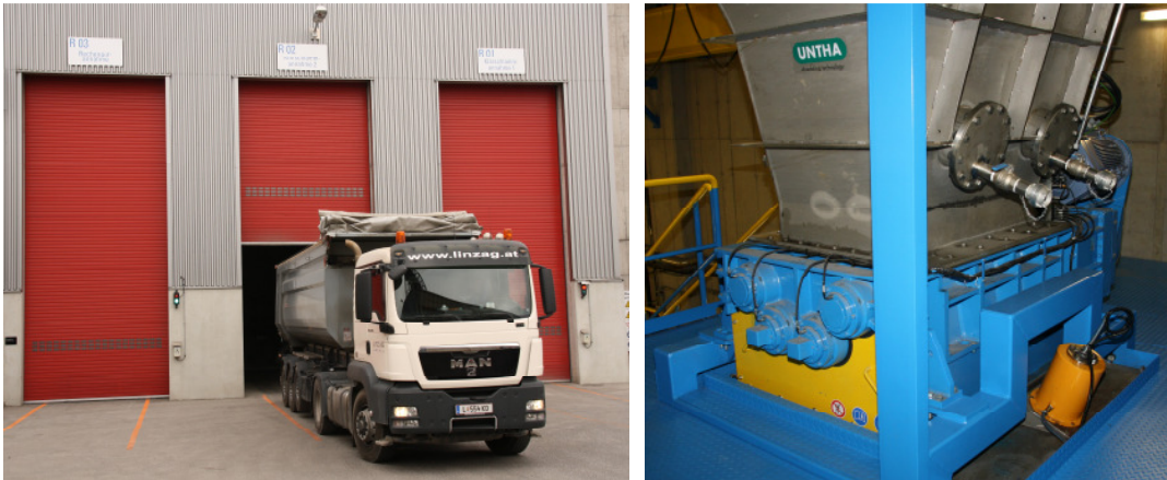
RHKW Linz Screening residues line: Separate reception hall with air control and shredding machinery with closed conveying
