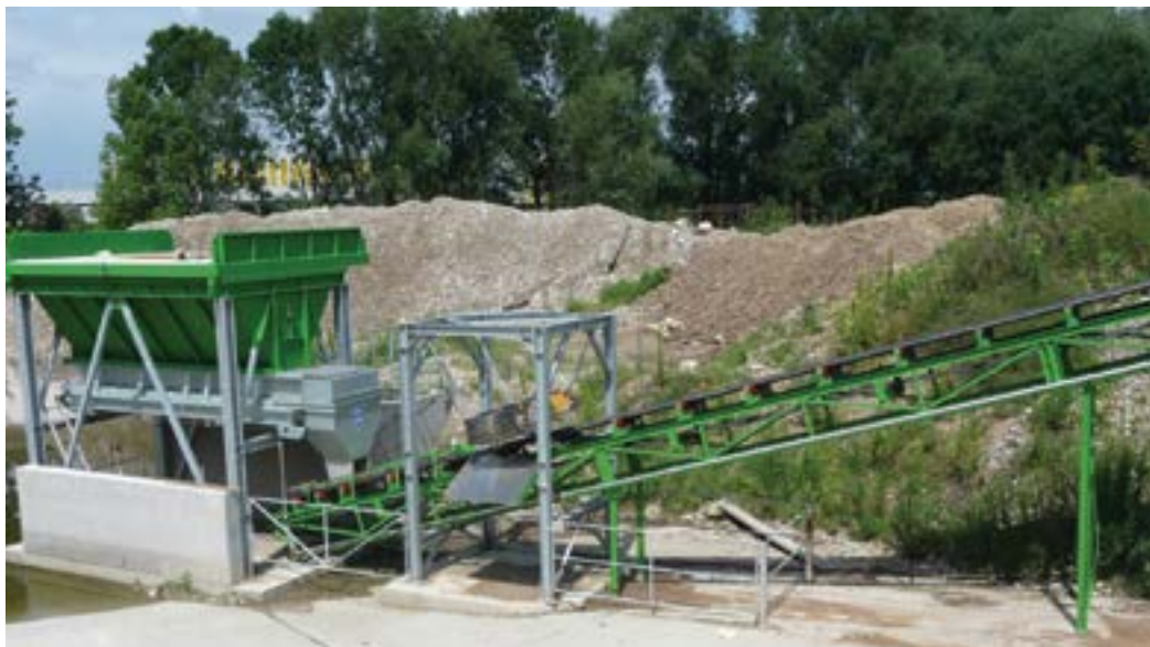
Figure 69: Soil treatment plant
