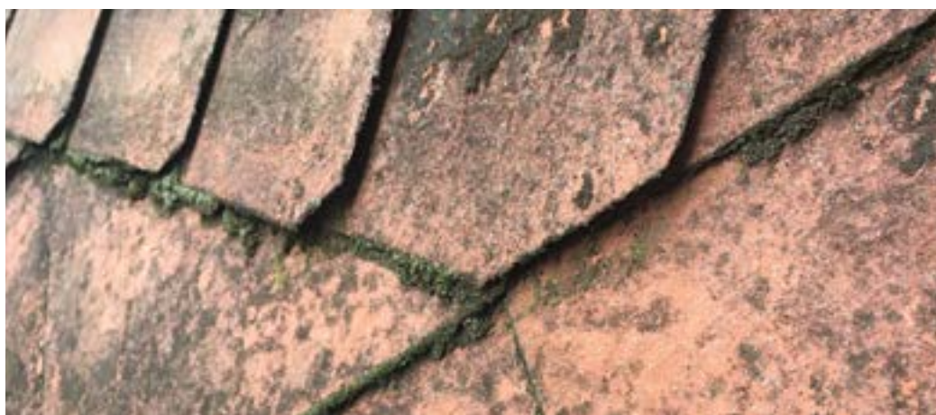
Figure 44: Roof shingles containing asbestos
