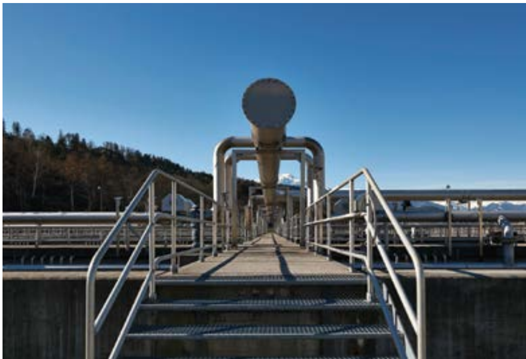
Figure 114: Waste water purification plant
