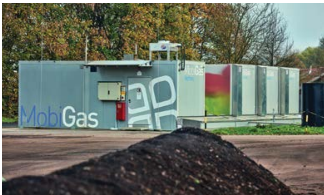
Figure 61: Mobile biogas plant
