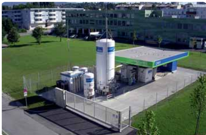
Figure 1: HyCentA facility (Hydrogen Center Austria)
